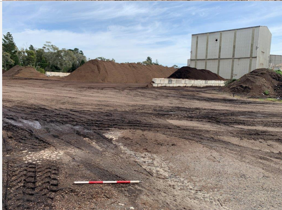
Plate 2: View of gravel pad and piles of soils and sand (Matthew Barker 8/10/21) facing northwest
