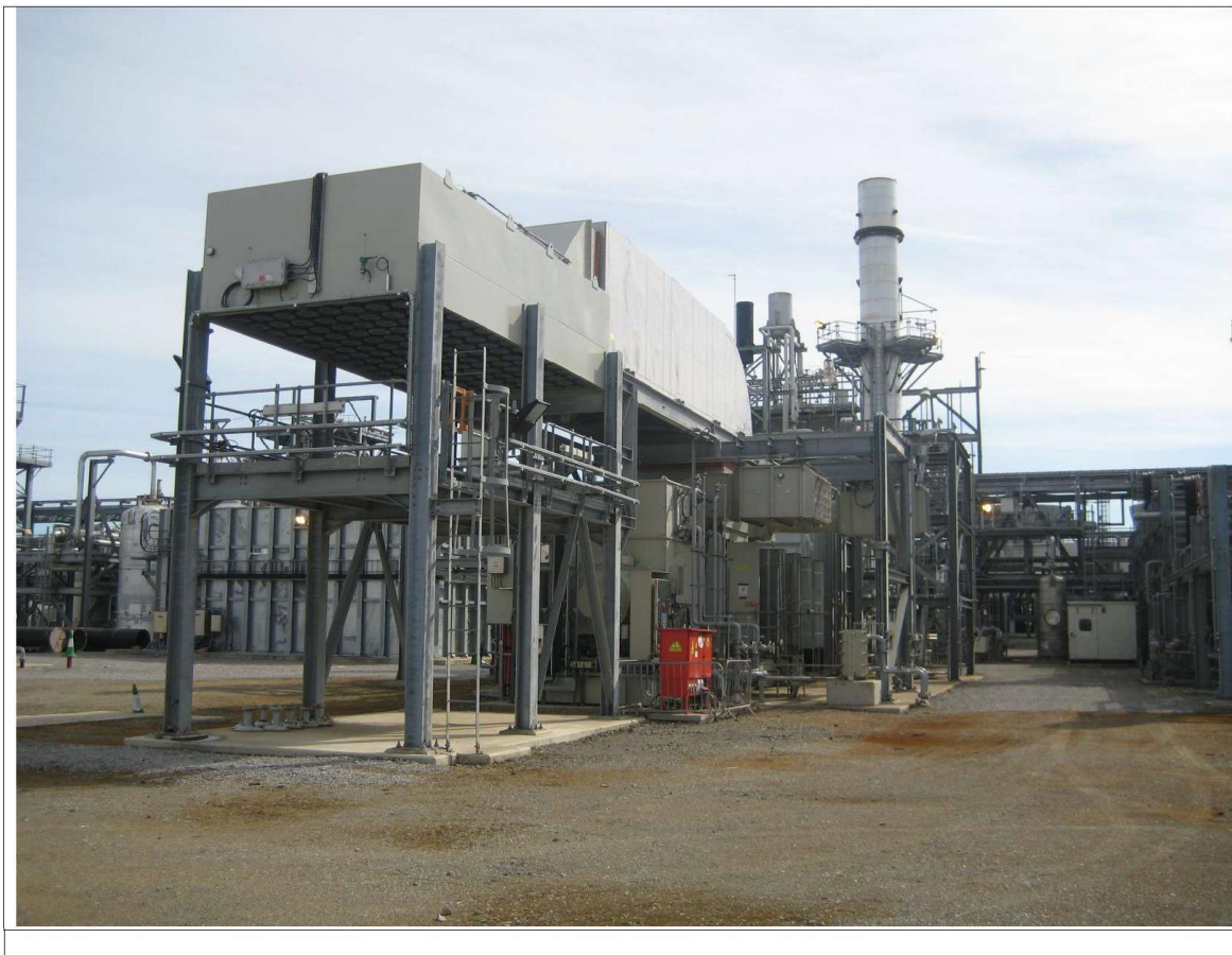
Solar Titan 130 gas turbine generator
