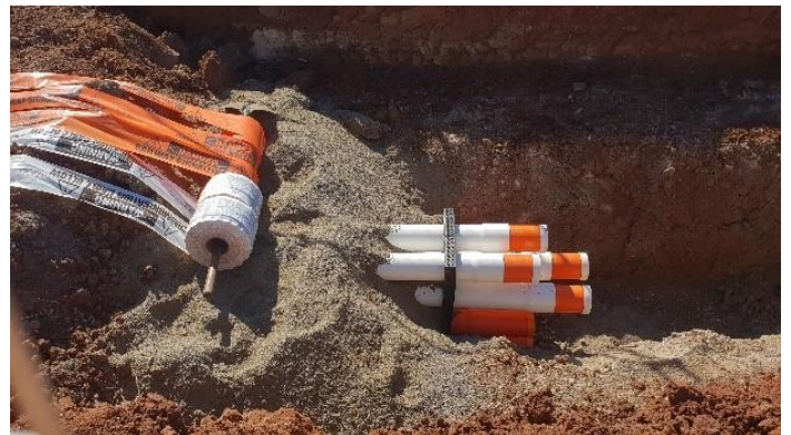
Glass sand, as per the Metro Trains Melbourne recycled glass specification, surrounding combined services conduits in a rail corridor Source: McConnell Dowell of the Western Program Alliance
