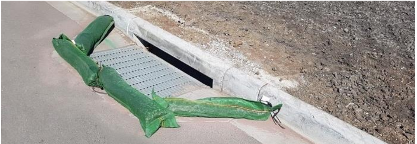
Figure 5.3. Silt sock in use to prevent sediment entering drain inlets (photo courtesy of McConnell Dowell).
