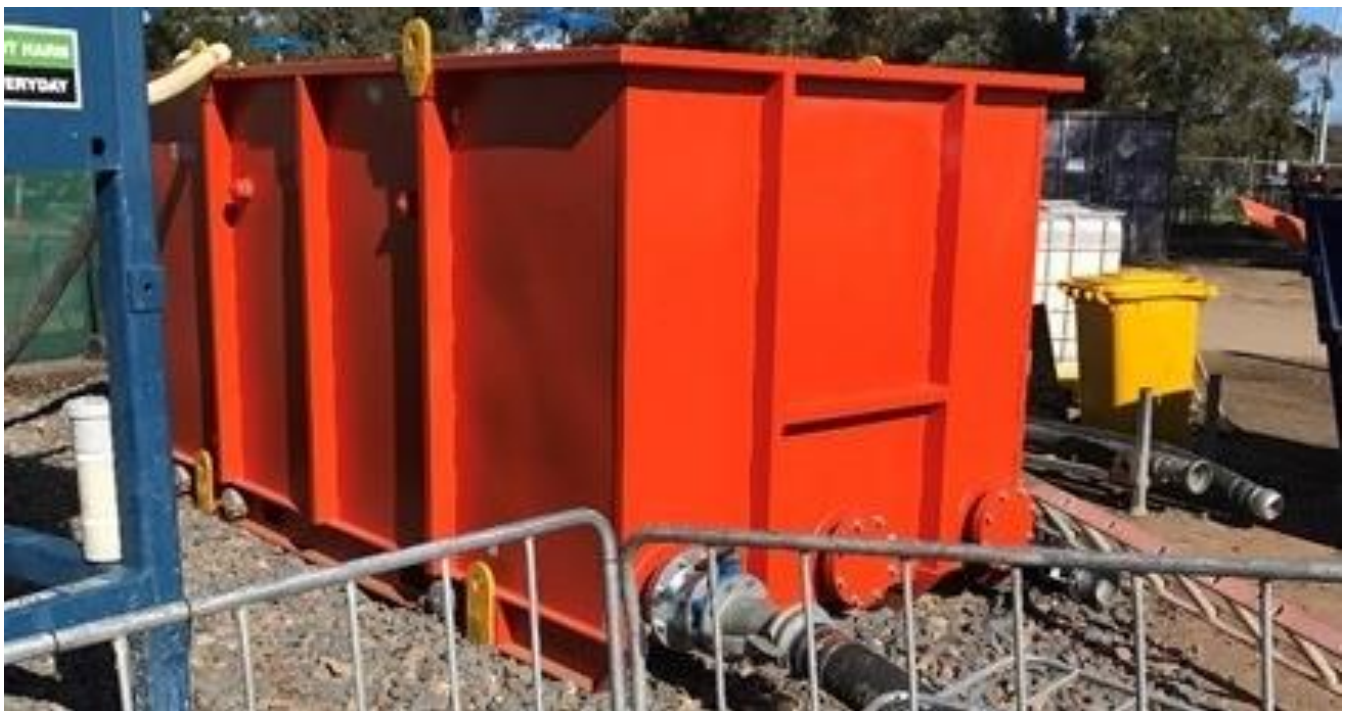
Figure 5.2. Portable sedimentation tank (photo courtesy of McConnell Dowell).
