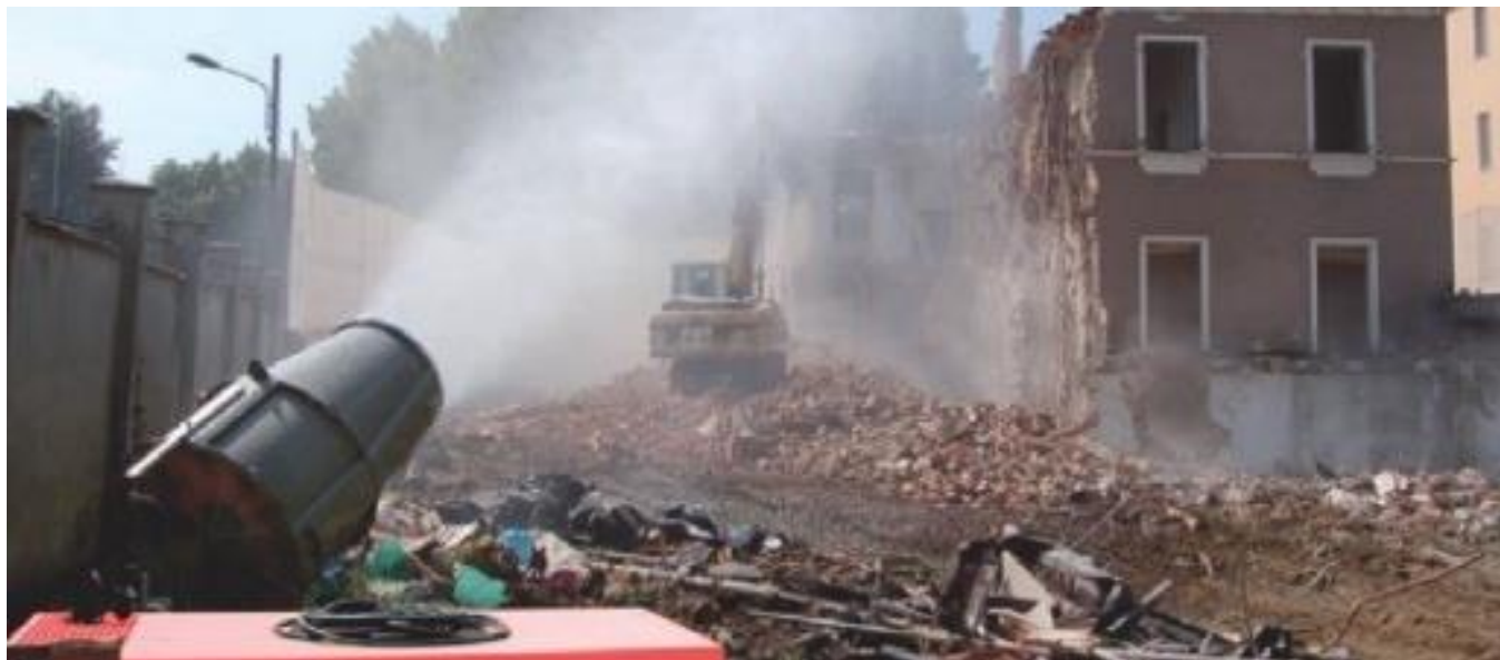
Figure 5.5. Dust suppression using water spray during demolition works (photo courtesy of Kane Constructions).
