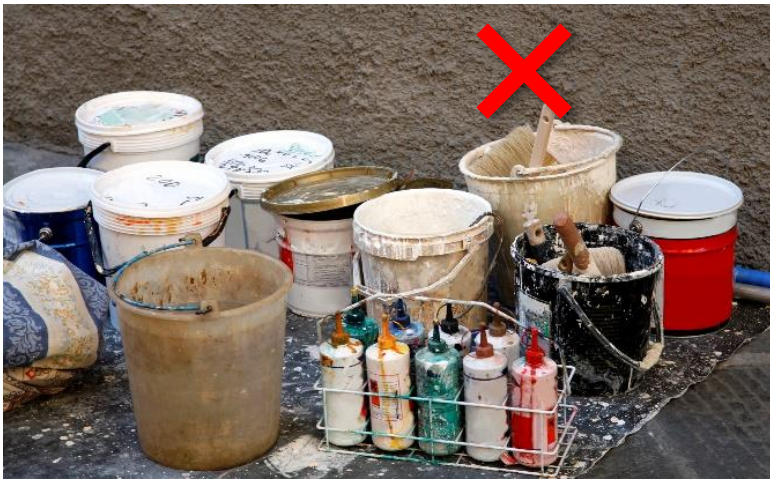
Figure 7.1. Incorrect chemical storage onsite.
