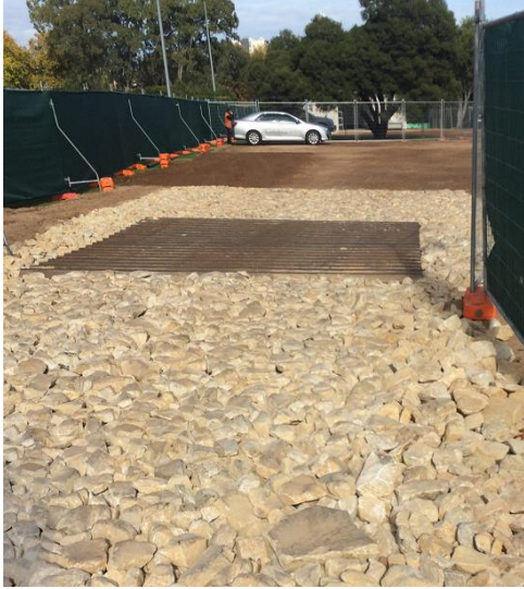
Figure 2. Rumble grid (photo courtesy of McConnell Dowell).
