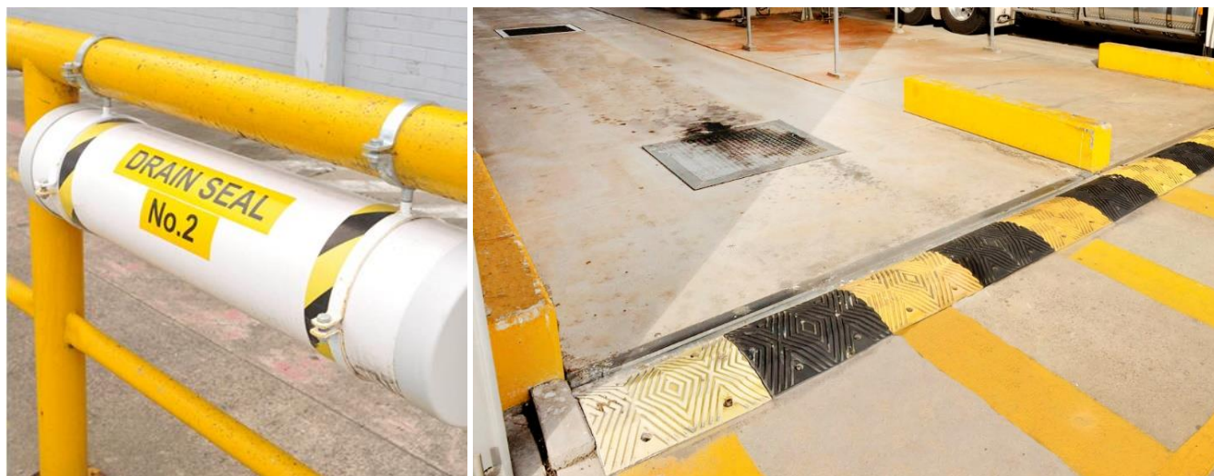
Figure 7.5. Drain seal (left) and rollover bund (right).
