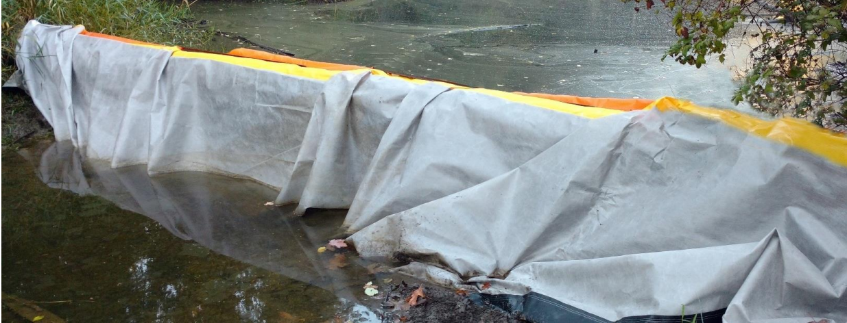
Figure 1. Engineered silt curtain installed to prevent migration of sediment for construction works within a waterway.
