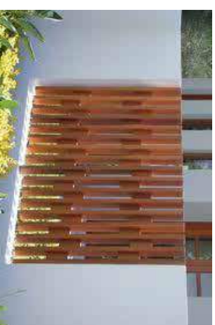
Image 6 Courtyard Fence Concrete panels with natural concrete render finish with timber battens screen inserts in client selected stain finish fixed to steel subframe
