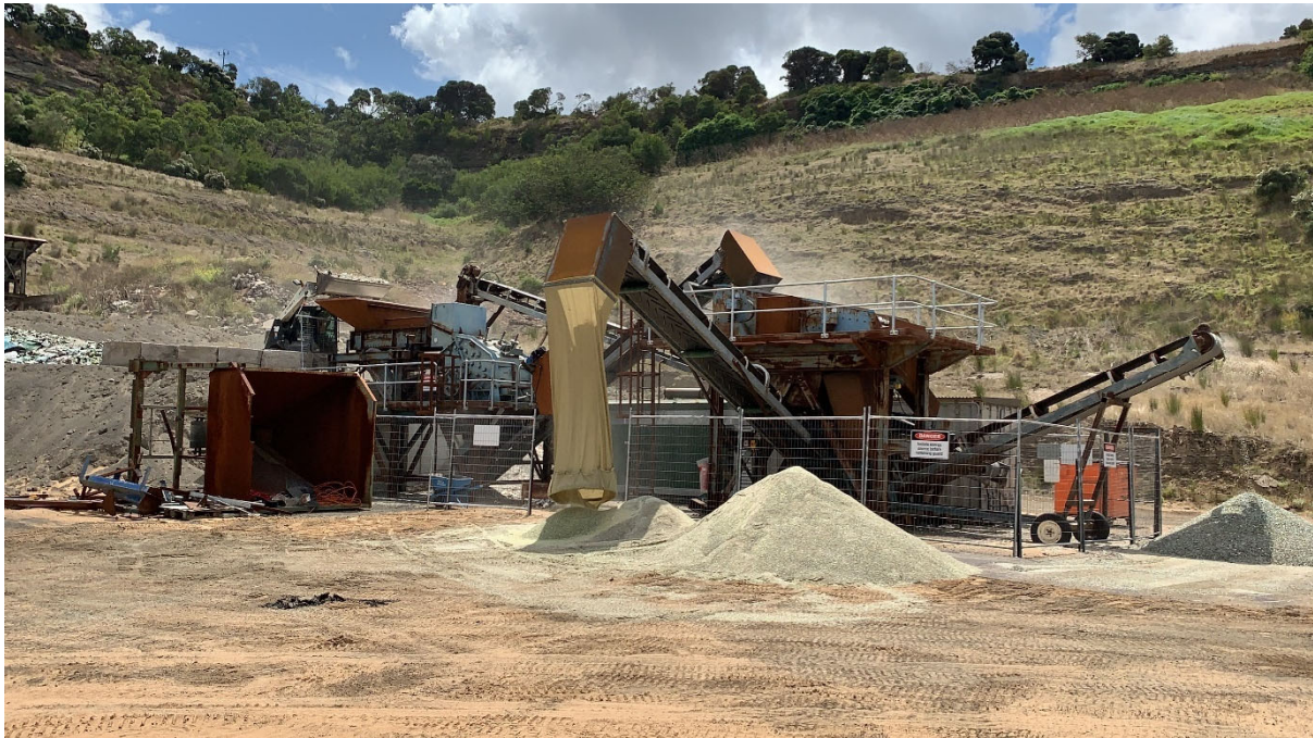
Figure 6-3 Photo of glass crushing and screening plant (in-situ at Koroit quarry)
