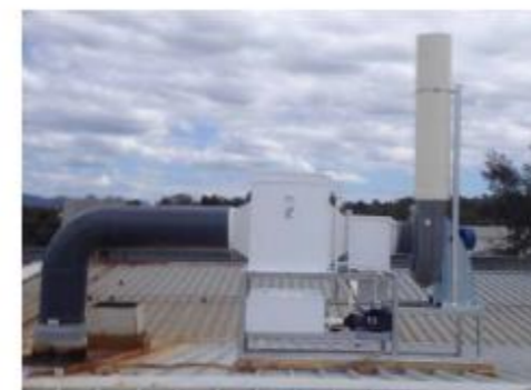
Roof mounted Advanced Air® fume scrubber 1200L/s.
