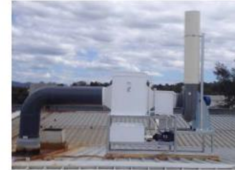
Roof mounted Advanced Air® fume scrubber 1200L/s.
