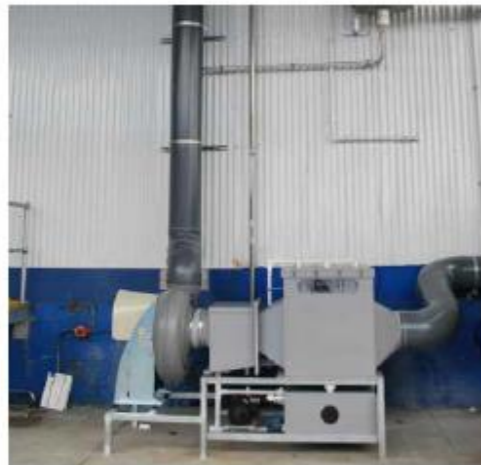
Advanced Air® fume scrubber 900L/s.
