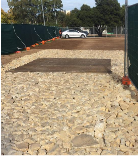
Figure 2. Rumble grid (photo courtesy of McConnell Dowell).
